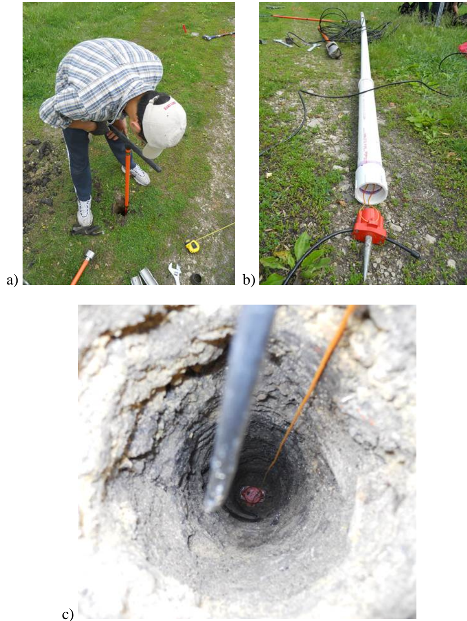
Figure 6.10 Borehole geophone preparation for MIBS field testing: (a) drilling borehole by hand-auger, (b) PVC pipe insertion device for borehole geophone, and (c) borehole geophone coupled to bottom of borehole by ground spike.
